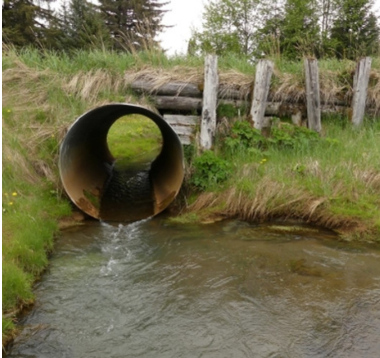
A perched culvert that's undersized passes Harry Hall Creek under a road in Gustavas, Alaska.
