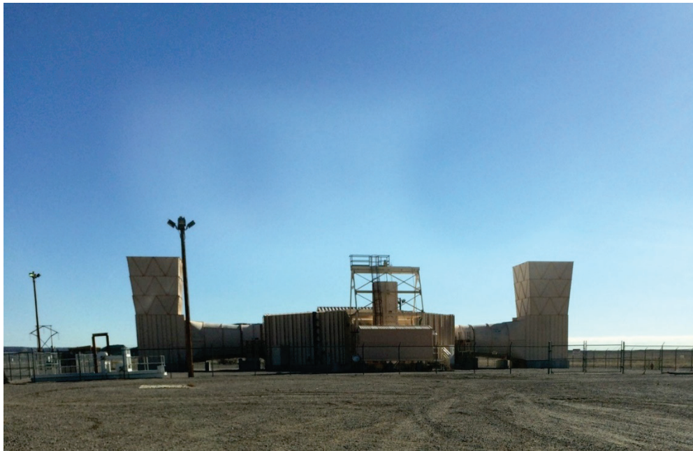
Figure 2.1-2: Photograph of Aboveground Ventilation System at the San Juan Mine
