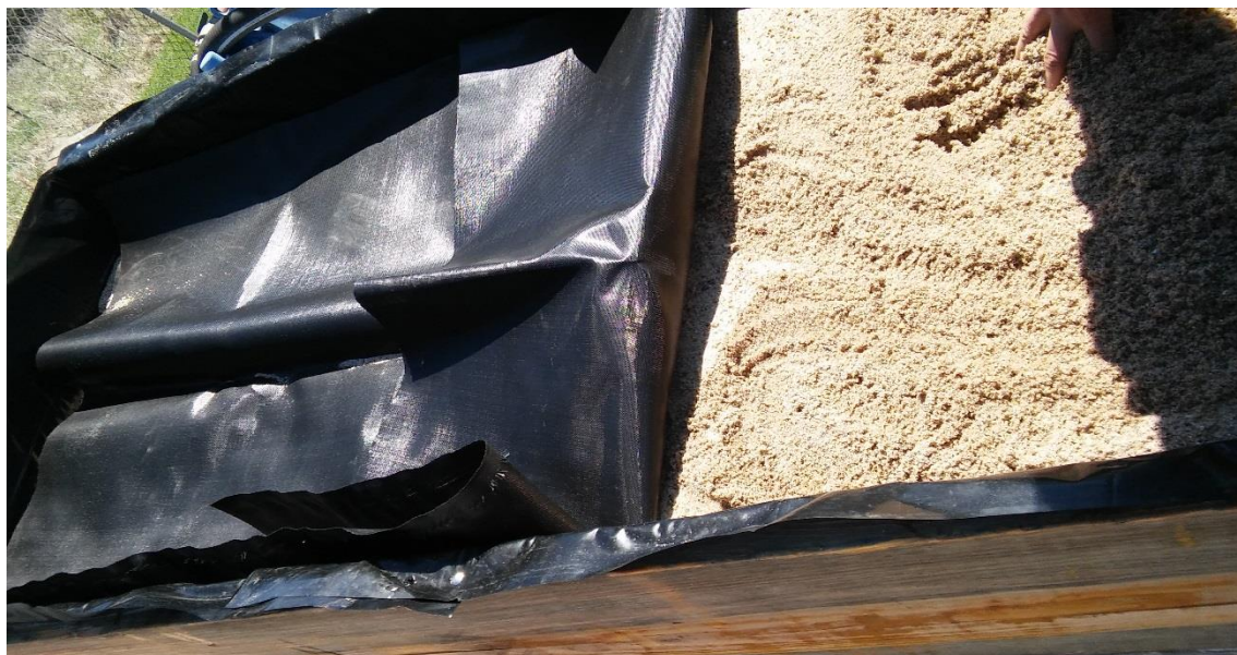
Figure T3.5 Placement of permeable geosystemic material as a divide between AMD soil treatment layer and free draining soil.
