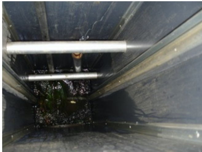
Figure 4.30. Agri-Drain flow control structure (view from above).
