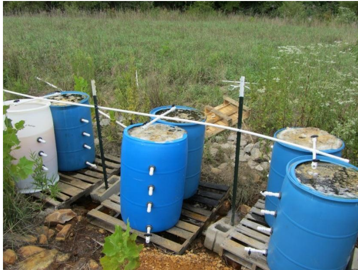
Figure 6: Photograph of reactors actively receiving AMD influent at the Tab-Simco AML site. A main PVC pipeline extends over the three pairs of reactors in which cross fittings allow AMD to be distributed in each reactor.
