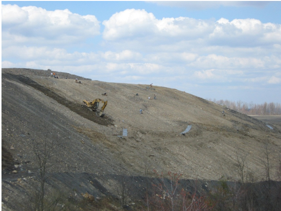
Figure 2-4 National site after the FRA reclamation process and during the construction of earthen berms. The tan sandstone surface layer can be seen in the surface materials to the right of the track hoe.
