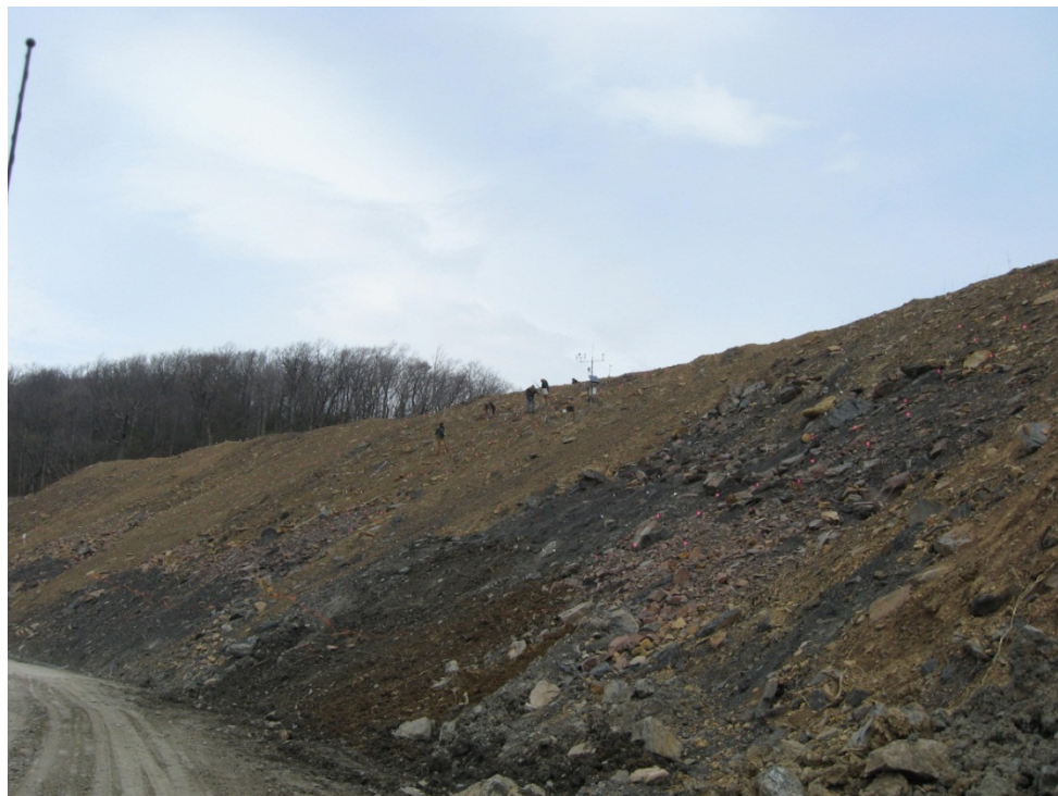
Figure 2-5 Premium site after the FRA reclamation process and during the installation of the weather station.
