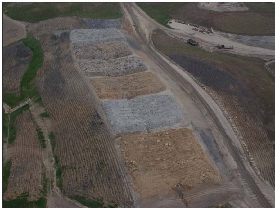
Figure 1-2 Pike County KY instrumented low compaction fill sites for examination of tree growth and monitoring of ground water chemistry (Angel et al. 2007); Barton et al. 2007).
