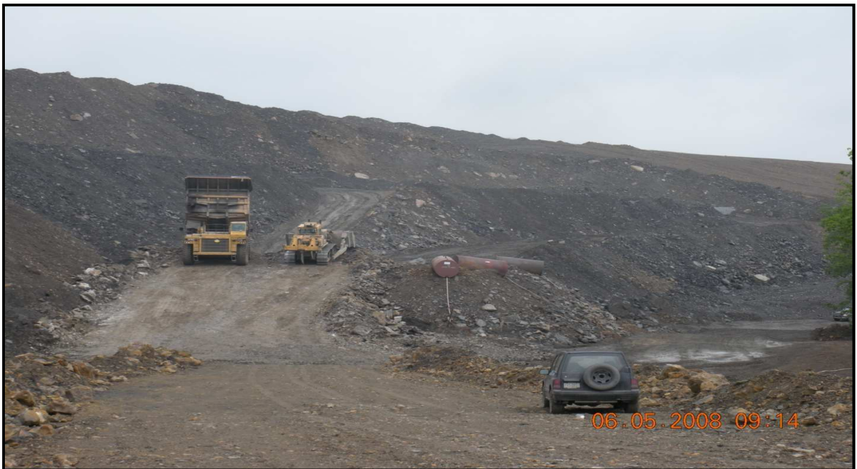
Figure 3.4: Active highwall elimination process using haulback at Brink Mine (B&M Energy), Pennsylvania
