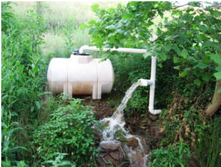
Figure 11. 300 gallon polyethylene tank with waste valve open
