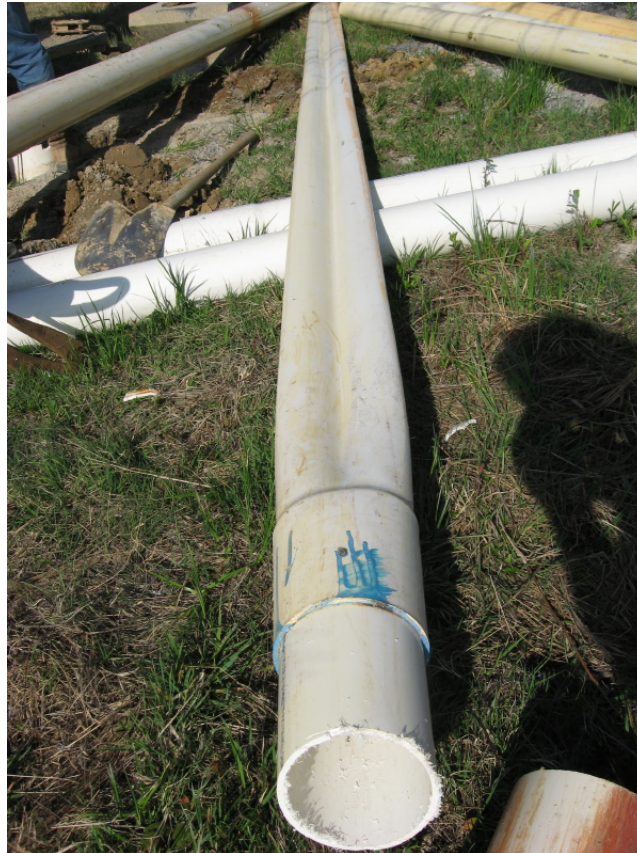
Photo 6. Crushed 5 inch casing
