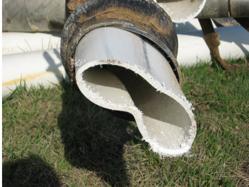
Photo 5. Collapsed 5 inch casing with shale trap.
