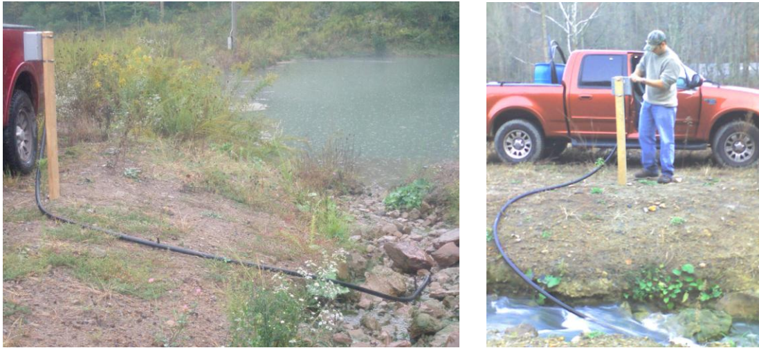
Figure 6. Installation of in-stream monitoring device.
