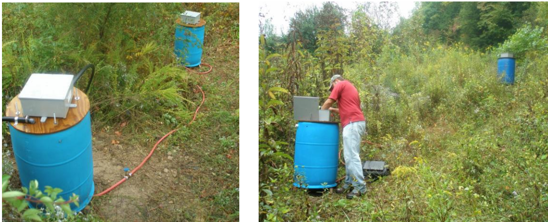
Figure 5. Installation of Apatite II treatment apparatus.
