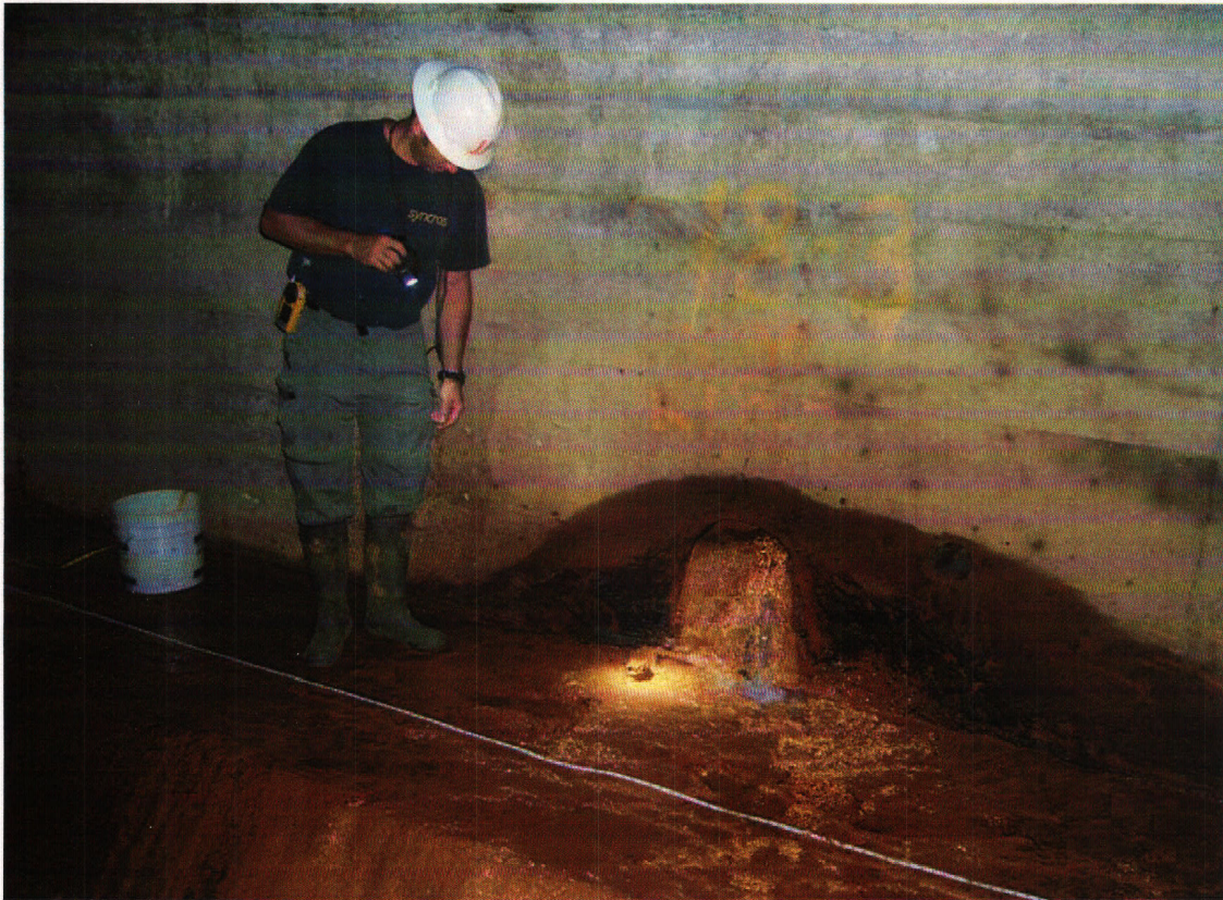
Figure 22: A 12" culvert in the 29 th St. tunnel is nearly plugged with AMD sludge.
