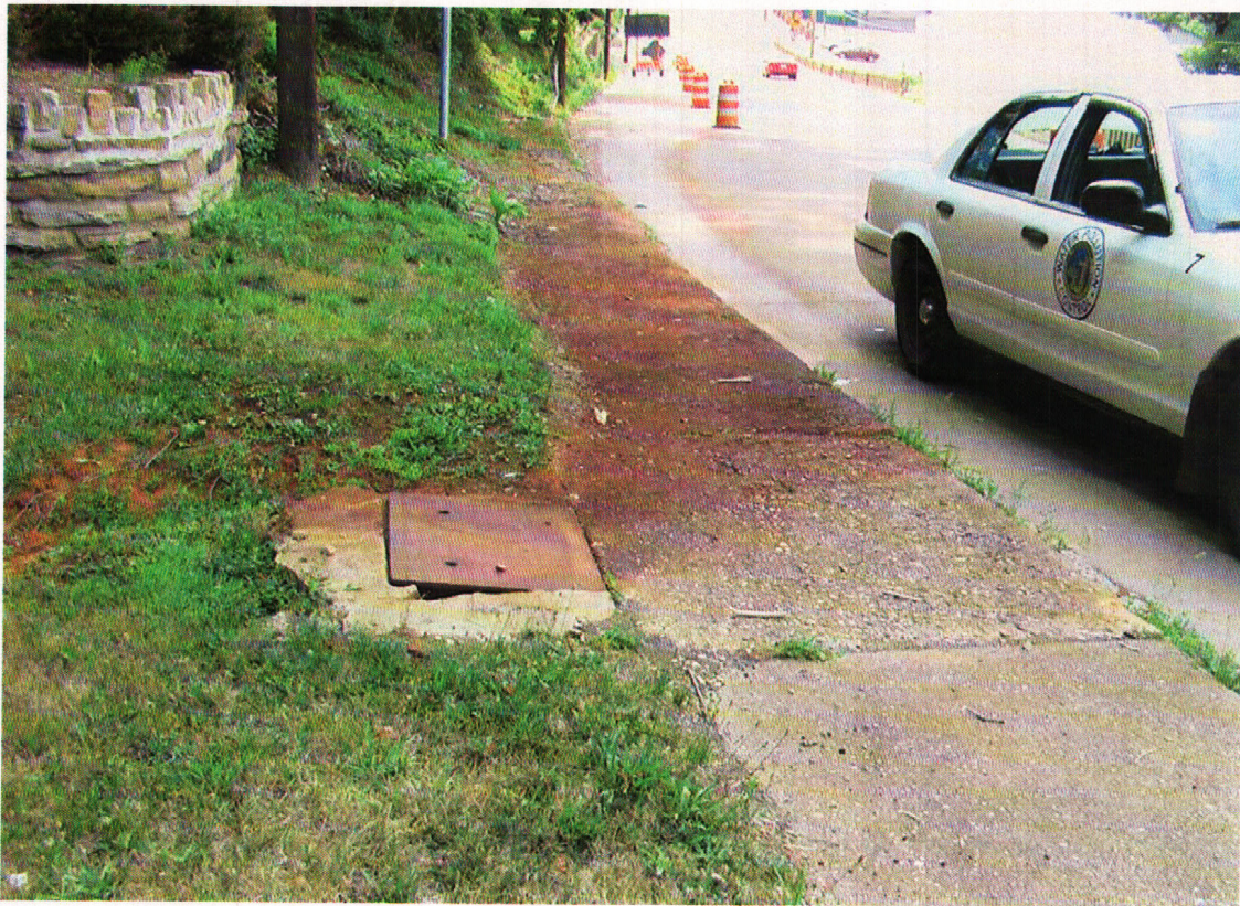
Figure 18: Wet-weather high flows are indicated by staining.
