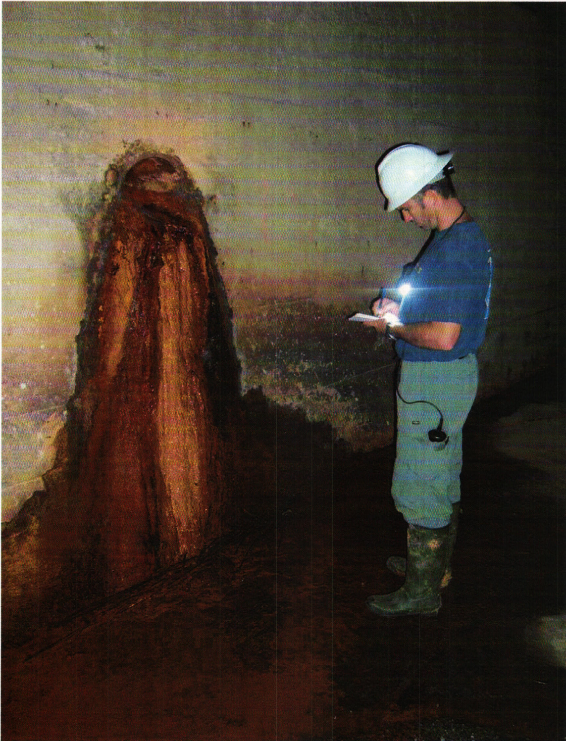
Figure 21: AMD sludge partially fills a 12" culvert in the 29 th St. tunnel.
