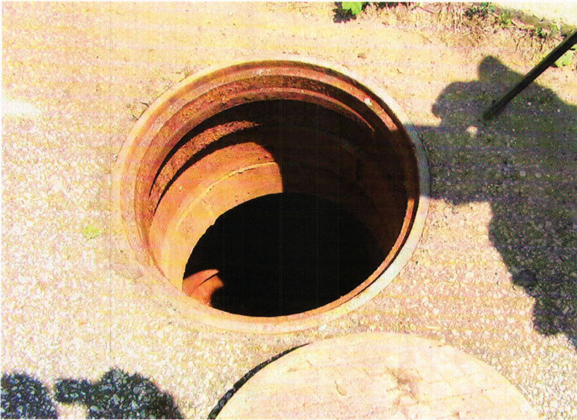
Figure 20: AMD sludge may plug sewer pipes causing overflow.
