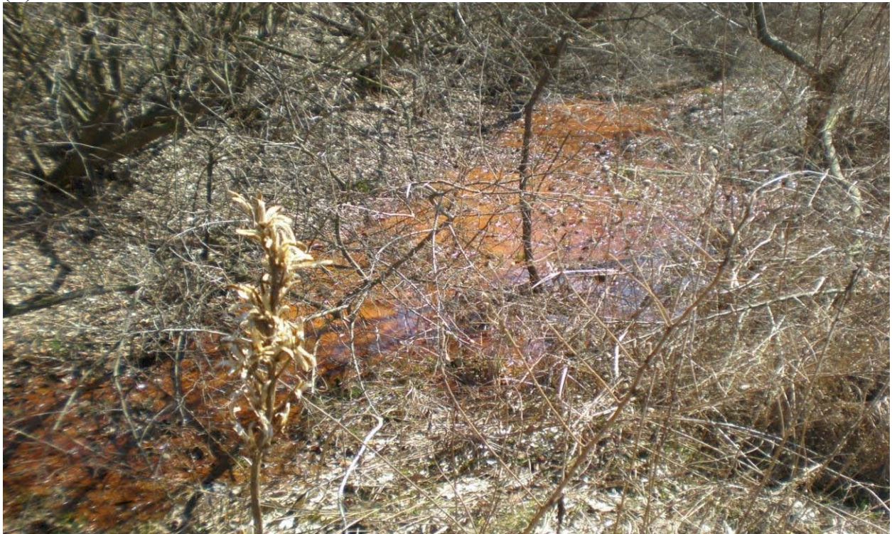
Fig. 8. (A) Start of new seep at UD-6c and (B) downstream view of UD-6c.
