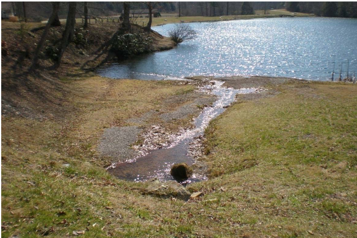
Fig. 3. Upstream seep UD-1 discharge into Black Creek Lake.
