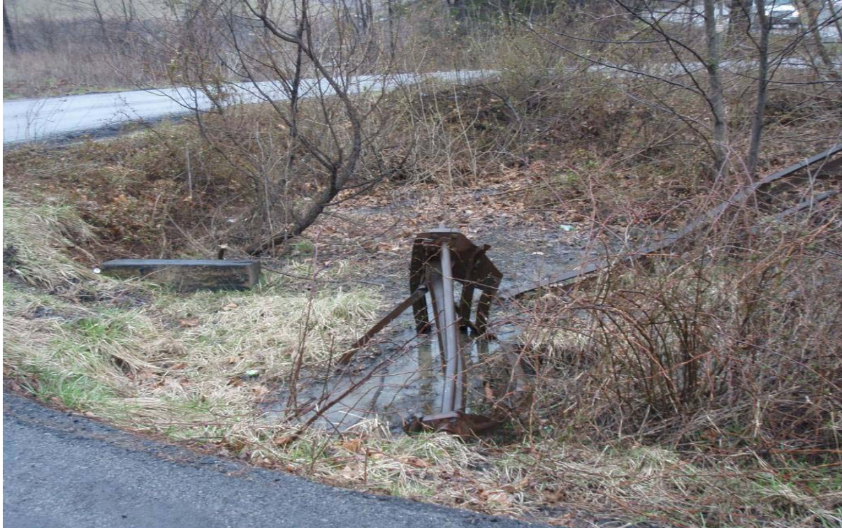
Fig. 17. Entry to culvert in center of vehicle turnaround near LBC-5. (Photograph provided by coal company personnel).
