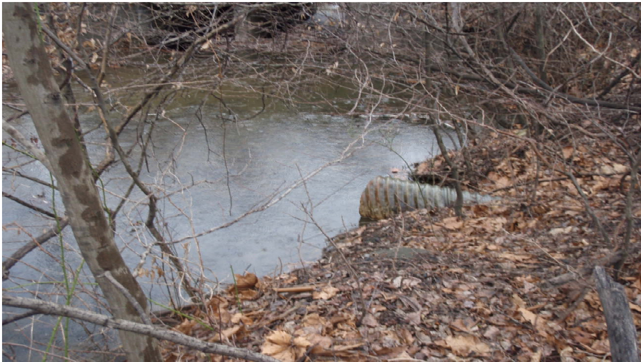
Fig. 18. Culvert that discharges runoff from vehicle turnaround to Black Creek near LBC-5 (photograph provided by coal company personnel).
