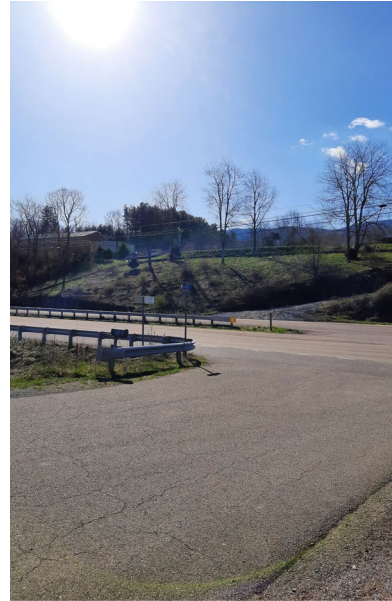
Jonah Rt. 19 access road in good shape
