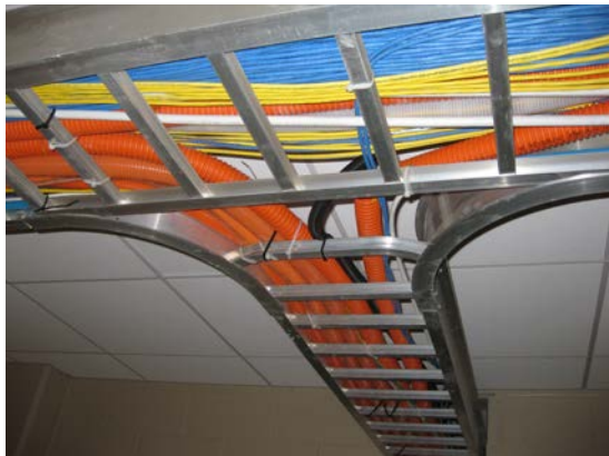
Communications Room Cable Trays Fairfax County Courthouse
