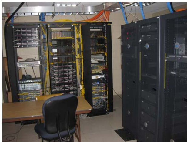
Computer Server and Communications Room, Fairfax County Courthouse
