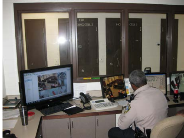
Isle of Wight Courthouse, Holding Area Control Room
