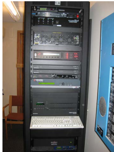
Dedicated Courtroom AV Closet, Fairfax County Courthouse
