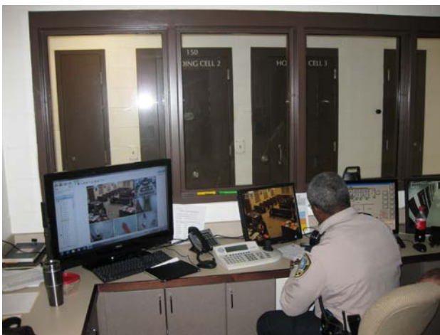
Isle of Wight Courthouse, Security Control Room
