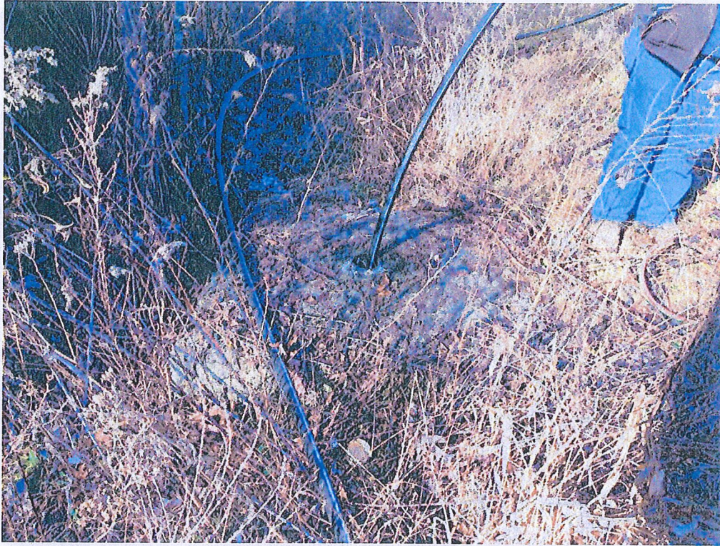
PHOTOGRAPH 1. View of groundwater monitoring well MW-3 being pressure grouted with a tremie pipe.
