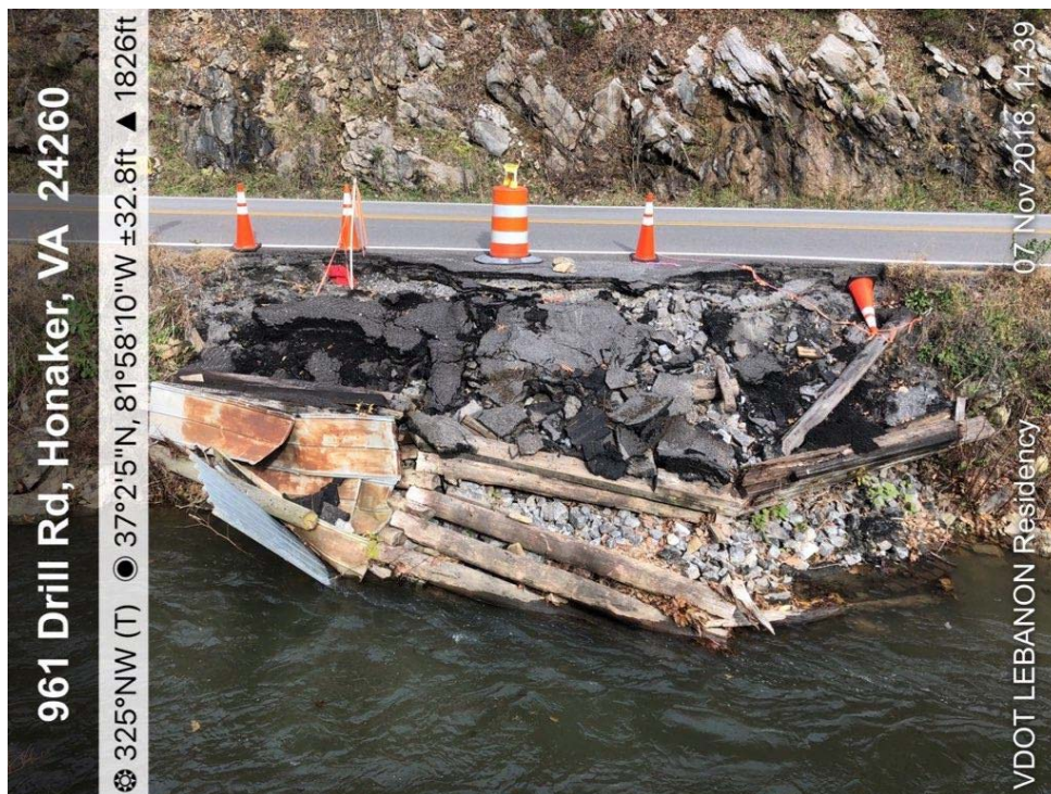
Photo 2: View of cribbing and other debris that will be removed before stream bank is stabilized. (11/9/18 by M. Bolling)
