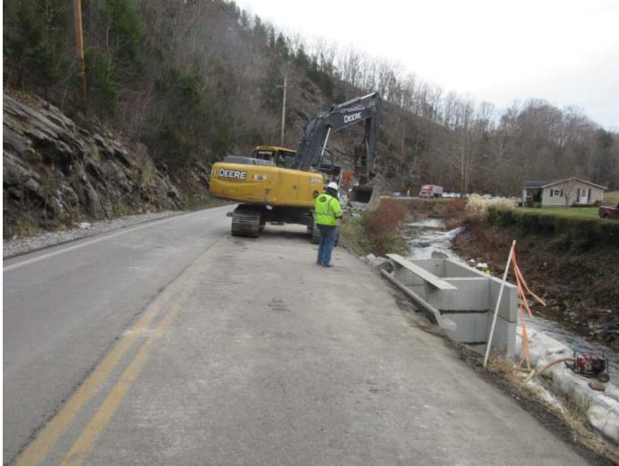
Photo 3: View looking south along Rt. 624 at roadway and bank/shoulder stabilization. (11/29/18 by M. Bolling)
