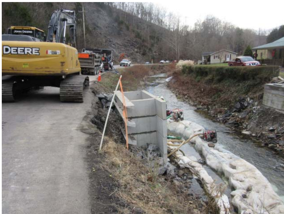
Photo 2: Another view looking downstream at evergreen retaining wall and dewatering operation. (11/29/18 by M. Bolling)
