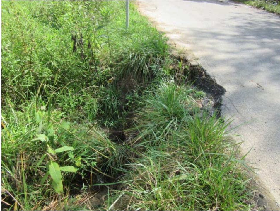
Photo 3: View of Culvert #1 inlet. The failing culvert is causing subsidence at the inlet end. 5 linear feet of Class 1 riprap will be installed to stabilize the inlet. (8/8/18 by E. Virts)
