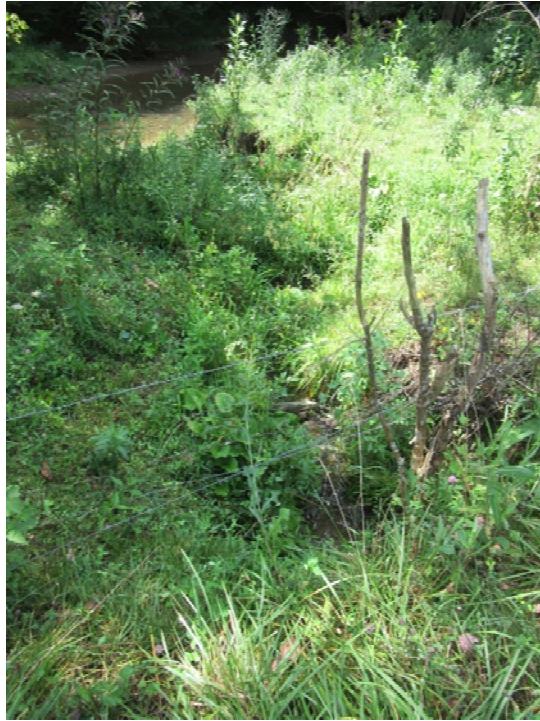
Photo 1: View looking downstream of Culvert #1, which is proposed for replacement. Copper Creek is approximately 30' from the culvert outlet. (8/8/18 by M. Bolling)
