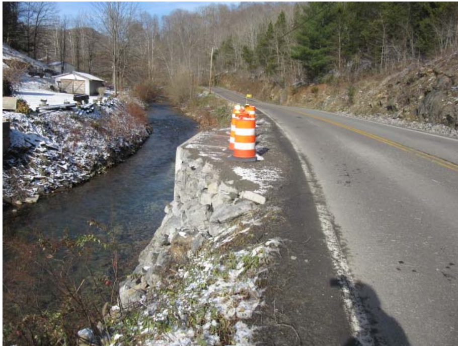
Photo 4: View looking north along Rte. 624 at stabilized stream bank/shoulder. (12/6/18 by M. Bolling)
