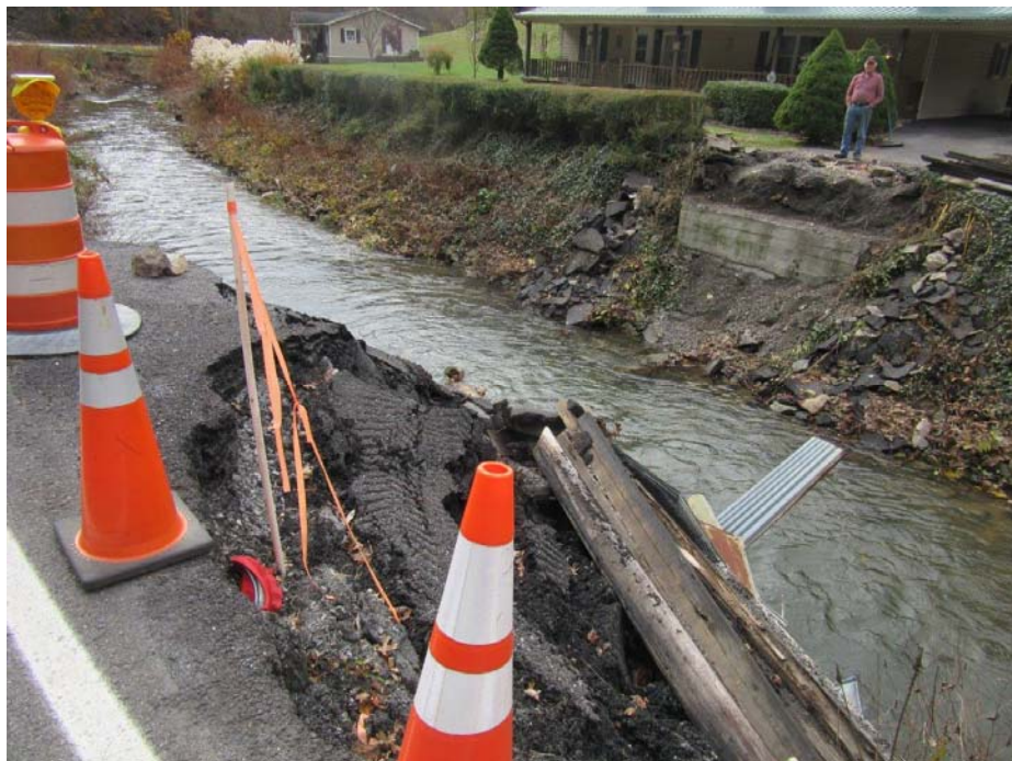
Photo 4: View of failing road shoulder (next to orange cones) that will be stabilized with an Evergreen retaining wall and Class II riprap. (11/13/18 by M. Bolling)
