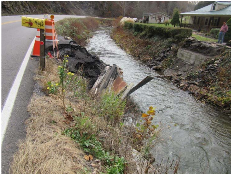
Photo 1: View looking downstream at failed private bridge and failing shoulder of Rte. 624. The loose debris will be removed and stabilized with an Evergreen Retaining wall and Class II riprap. (11/9/18 by M. Bolling)
