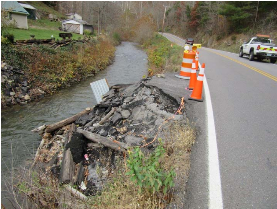
Photo 3: View looking upstream at failed bridge abutment and remaining debris. (11/13/18 by M. Bolling)
