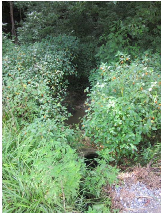
Photo 6: View of Culvert #2. 5 linear feet of Class 1 riprap outlet protection will be installed after the culvert end-section is repaired. (8/8/18 by M. Bolling)
