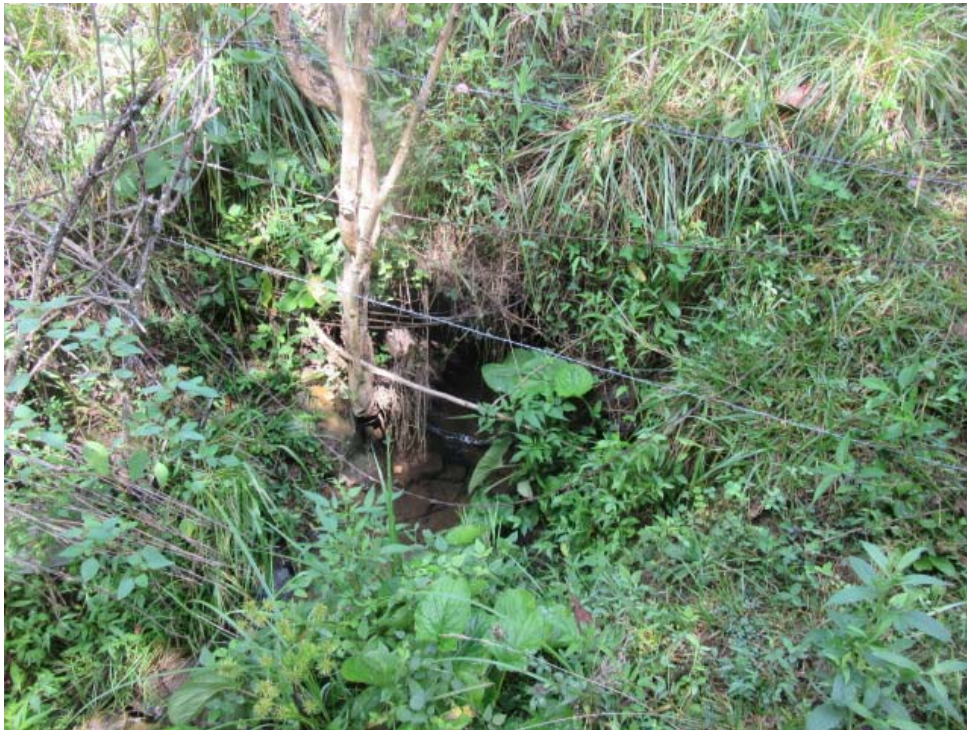
Photo 2: View of Culvert #1 outlet. 5 linear feet of Class I riprap outlet protection will be installed. (8/8/18 by M. Bolling)
