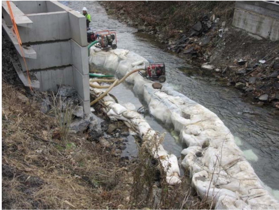
Photo 1: View looking downstream at dewatering operation and bank stabilization. (11/29/18 by M. Bolling)
