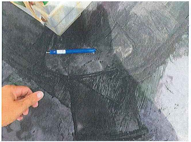
Hole in the curb flashing
