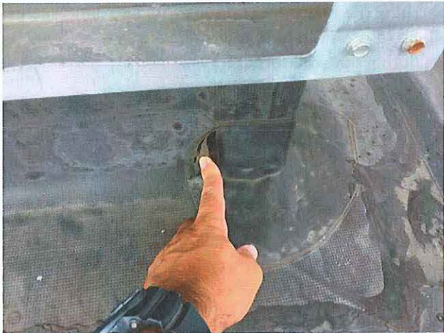
Opening in the top of a curb flashing
