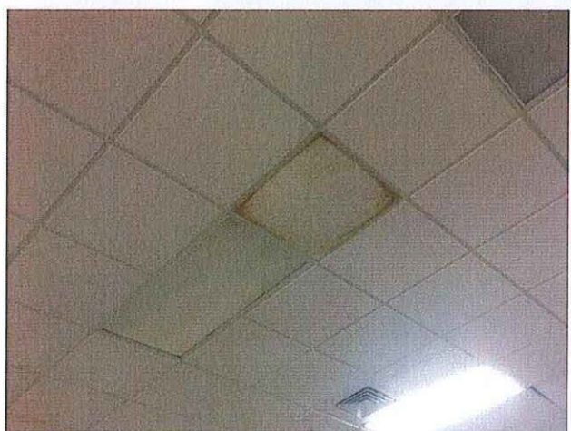
Interior picture of leak area
