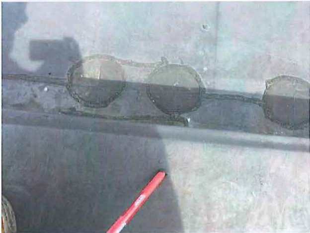
Hole in the field of the roof
