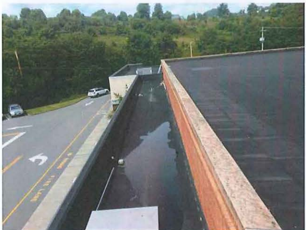
Drain area needs cleaned to reduce ponding water
