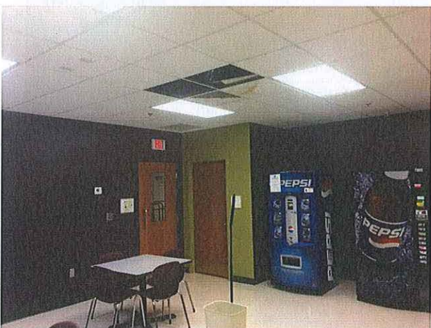
Interior picture of leak area
