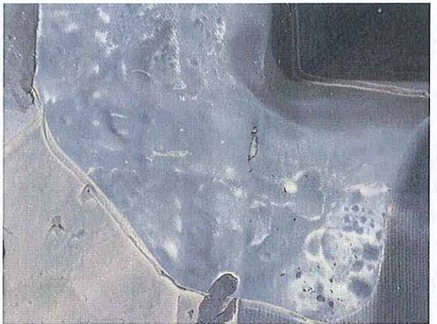
Split in the curb flashing
