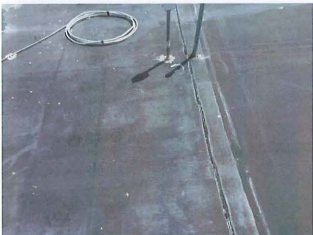
Pipes where caulking has failed
