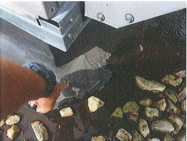
Split in the curb flashing
