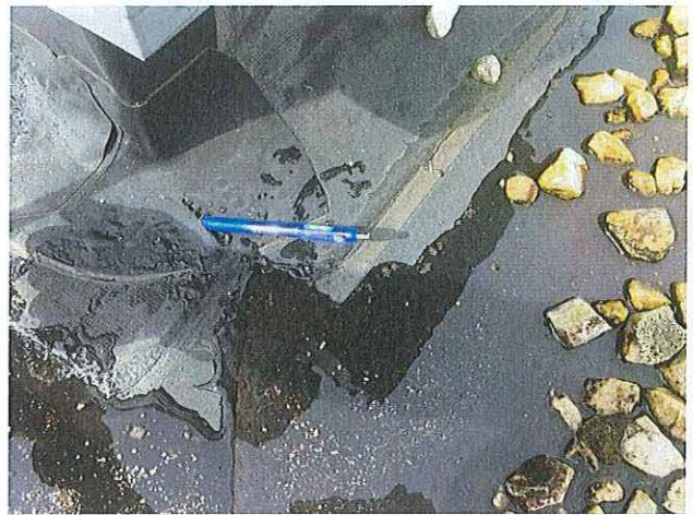
Split in the curb flashing
