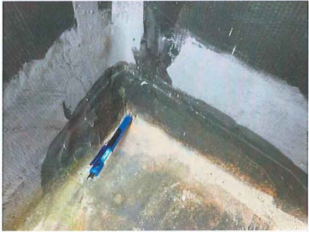
Hole in the corner flashing
