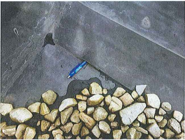
Opening at the seam at the expansion joint
