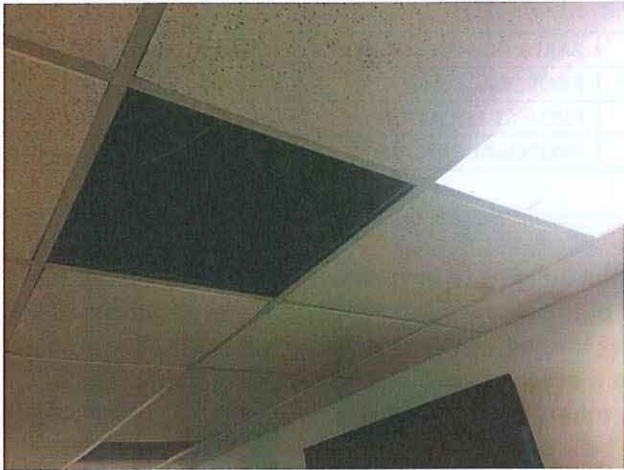
Interior picture of leak area
