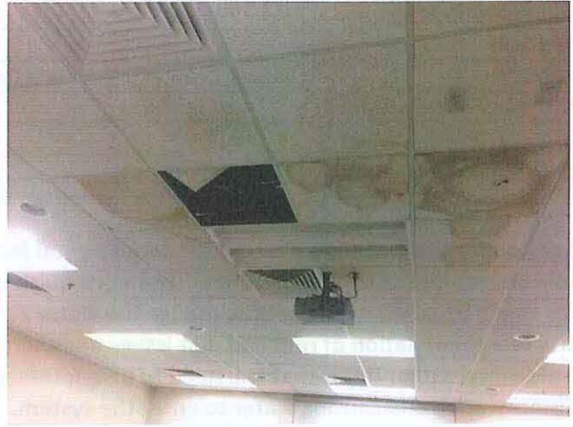
Interior picture of leak area
