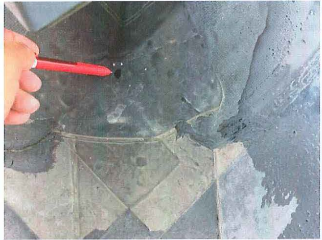
Hole in a curb flashing
