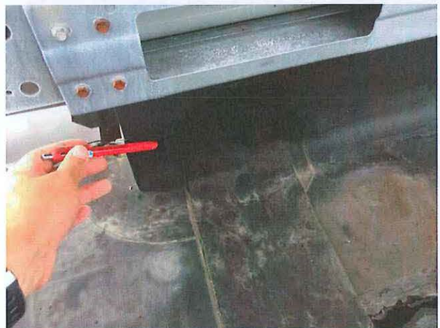
Split in the top of a curb flashing
