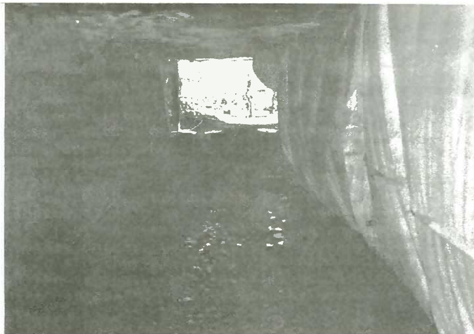
No. 5 View from waterhole looking outside showing line curtain and ventilation tubing
