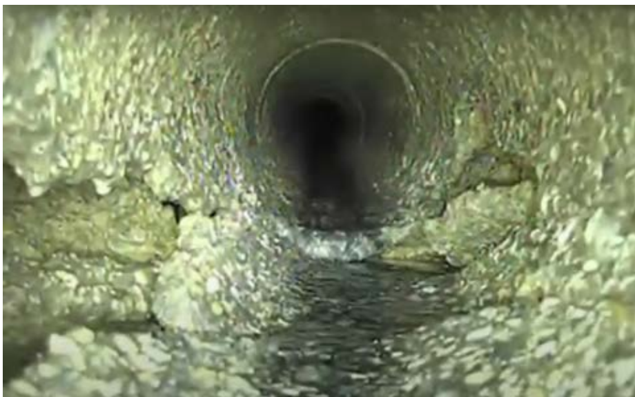
Figure 3.4.1 – Deteriorated Section of Concrete Sewer Line
