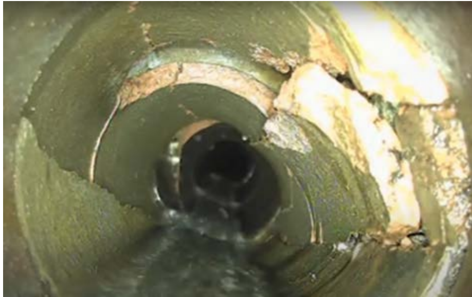
Figure 3.4.2 – Collapsed Section of Terracotta Sewer Line
