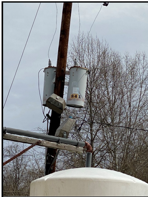
Figure 29: Old Scale House – Pole Mounted Transformers of Unknown PCB Content
