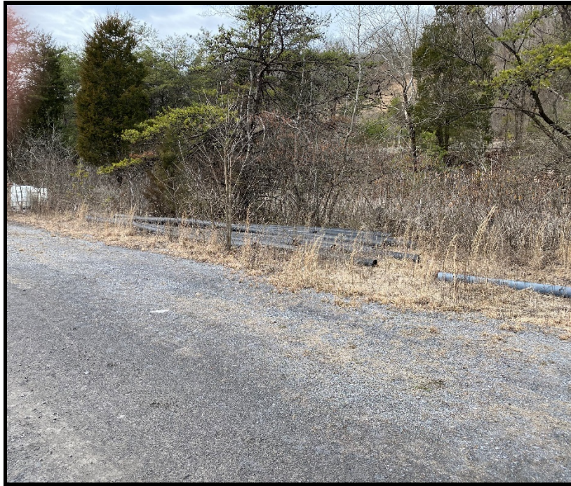
Figure 37: Access Road – General Debris (2 of 2)
