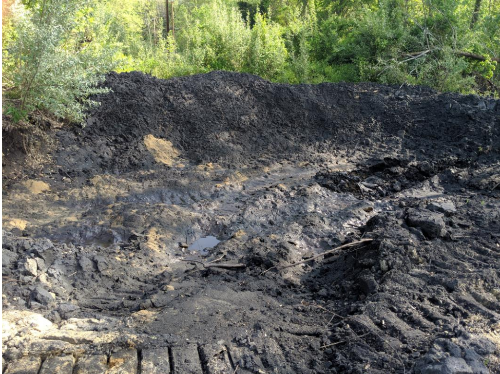
An area located near the building site that had been excavated to solid prior to backfill placement.
