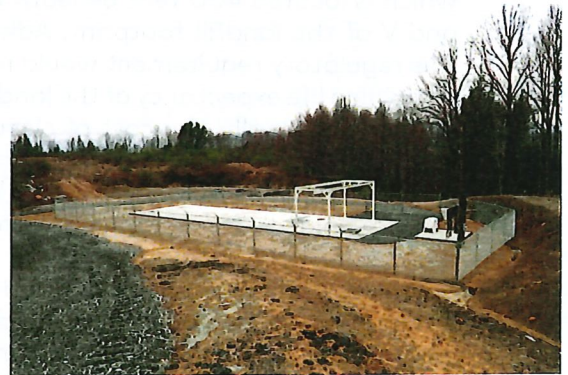
Leachate Pump Station - 2011
