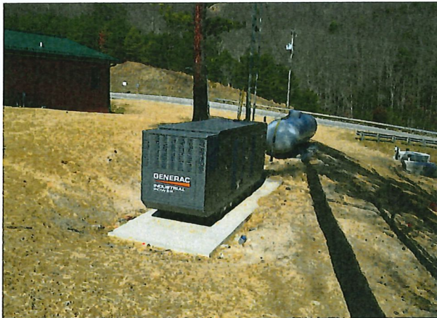
Completed New River Resource Authority Administration Building Generator
