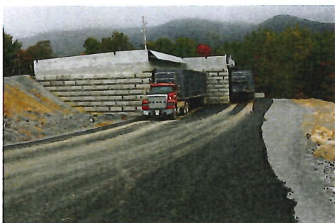
Tazewell County Landfill Solid Waste Convenience Center
