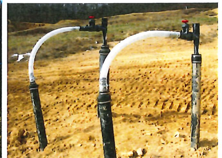
Tazewell County Landfill Gas Collection
