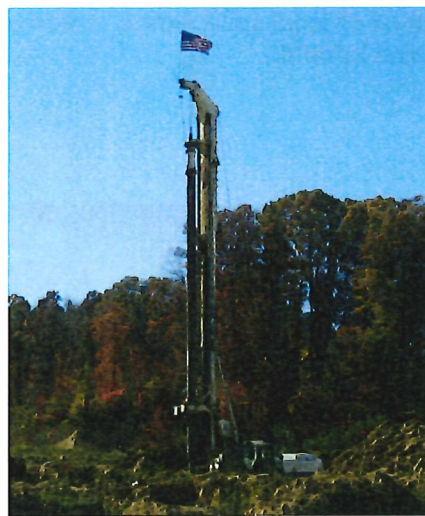
Tazewell County Landfill Gas Collection
